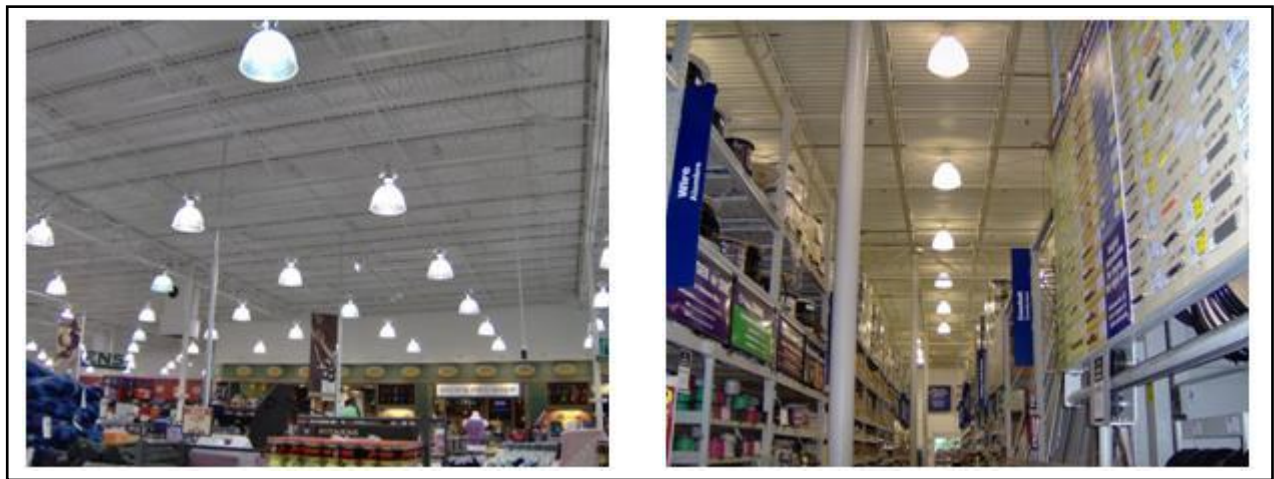
Figure 2: Typical high bay installations
